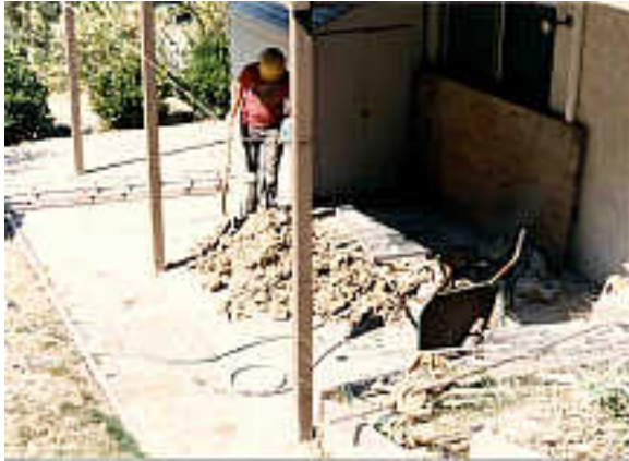
Figure A-1 Difficult cleanout location near the house
