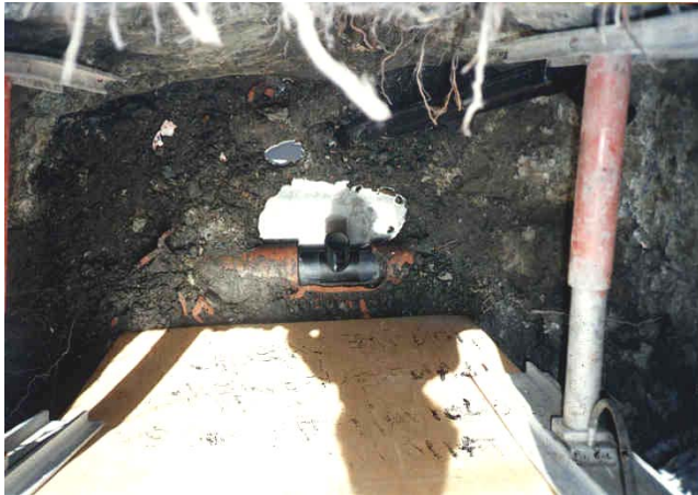
Figure A -9 Mainline Tee ready for lateral connection (a view from above)
